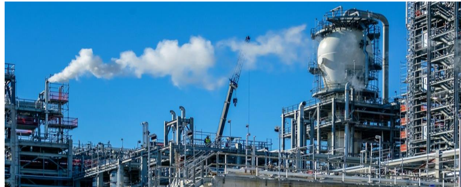
LLDPE – Purification Area with Reactor
