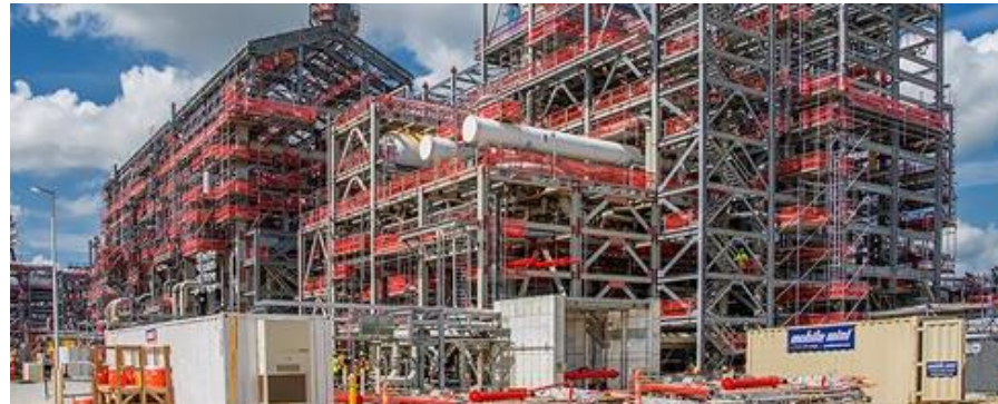
Cracker compressor house
